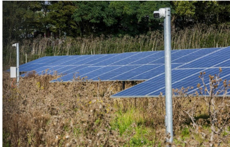
Image 9: Pole-mounted Security Camera
