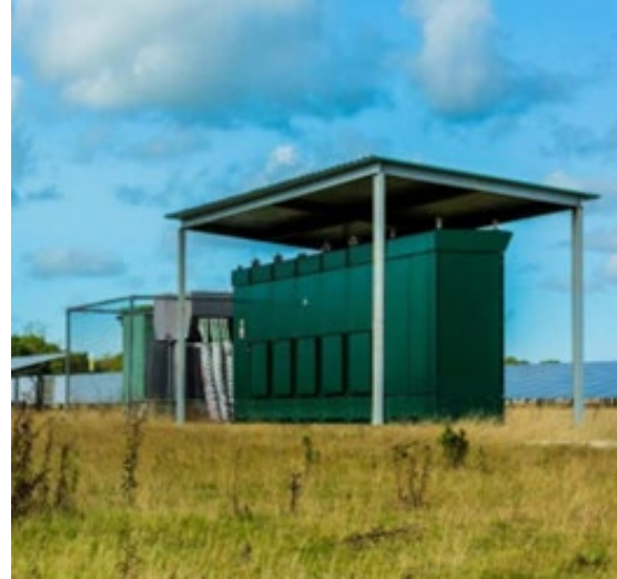
Image 4 Central Inverter Unit
