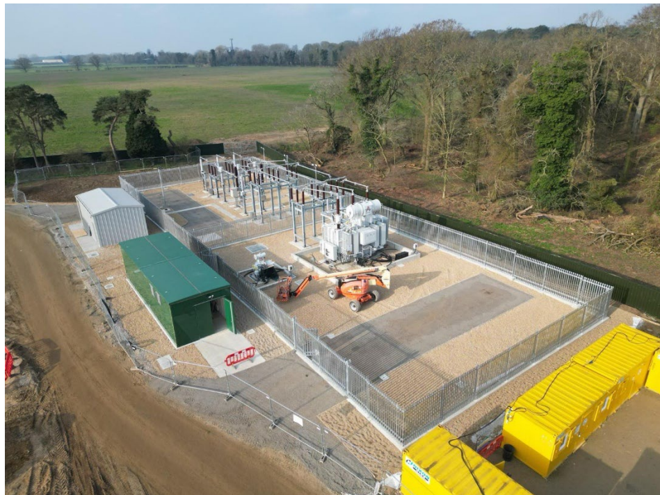
Image 5 132/33kV Substation (single transformer)
