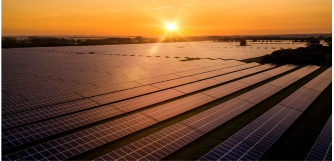
Image 2 Fixed South Facing PV Arrays
