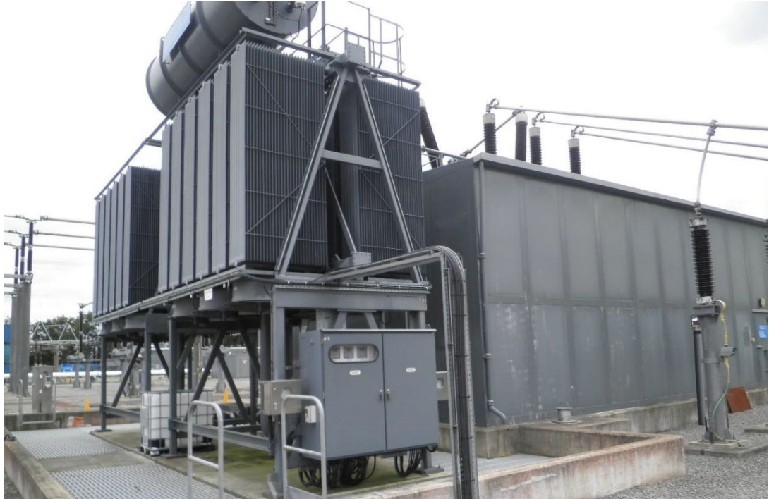
Image 6 Typical 400kV power transformer
